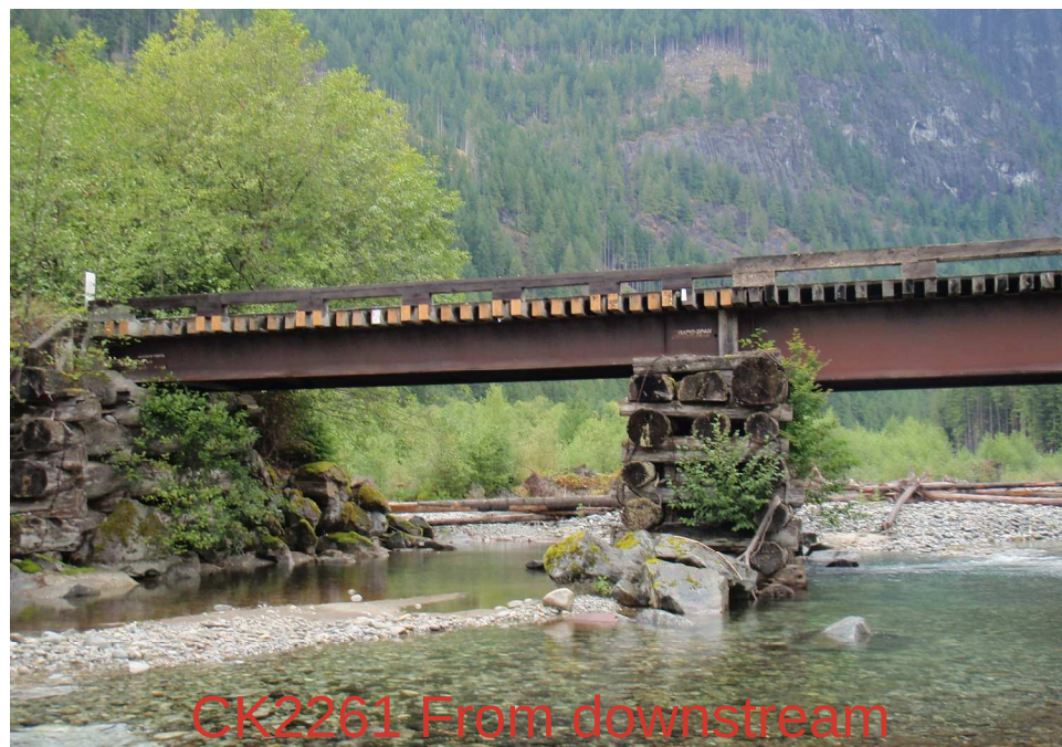
CK2261 Damaged deck
